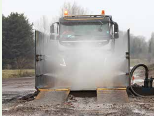
The contractors have been working hard throughout the bad weather to minimise the impacts of the work, with wheelwashes, checks at the construction access and traffic marshalls in place to minimise impact on local roads.
